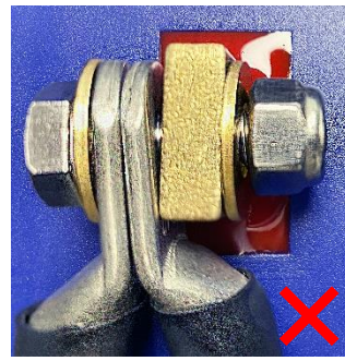
Improper connection for two lugs, top view
