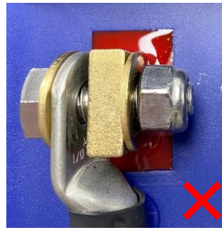
Improper connection for a single lug, top view
